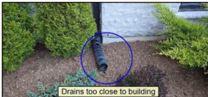
5. Discharge too close to building
