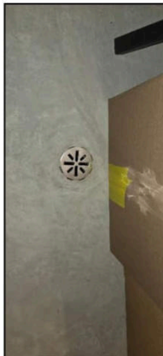
60. Near heating system
