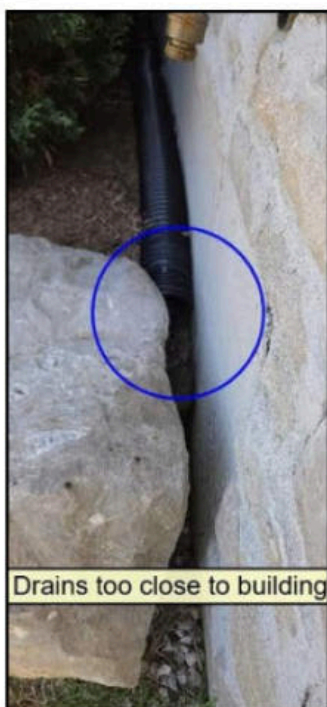
6. Discharge too close to building
