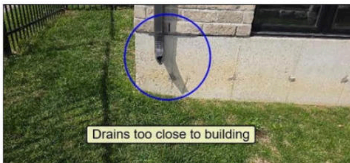
8. Discharge too close to building
