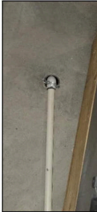
43. Discharges through floor slab
