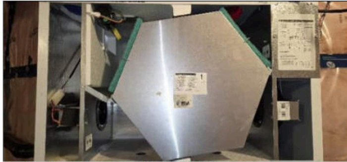
41. Heat recovery ventilator (HRV)
