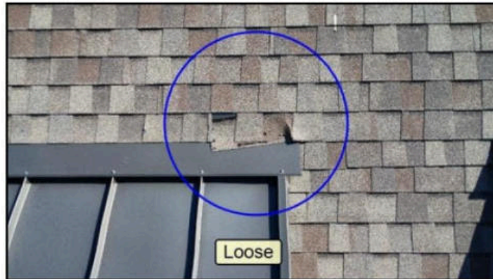
2. Missing, loose or torn
