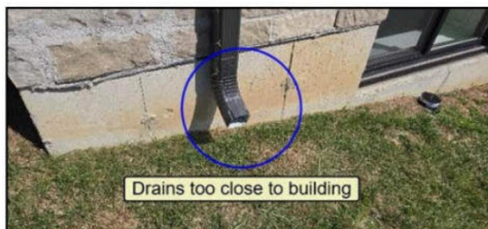
7. Discharge too close to building
