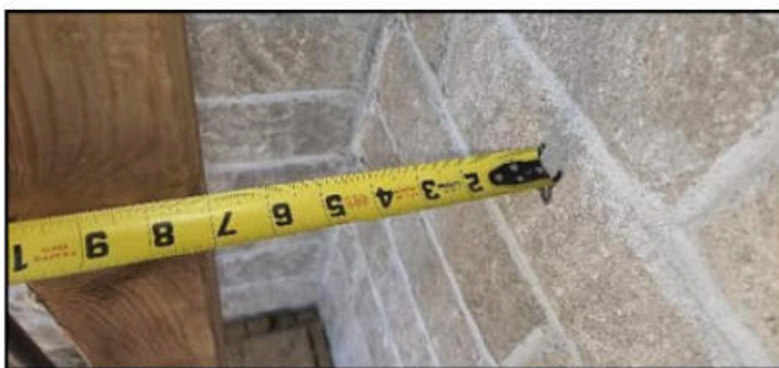
12. Spindles (balusters) too far apart
