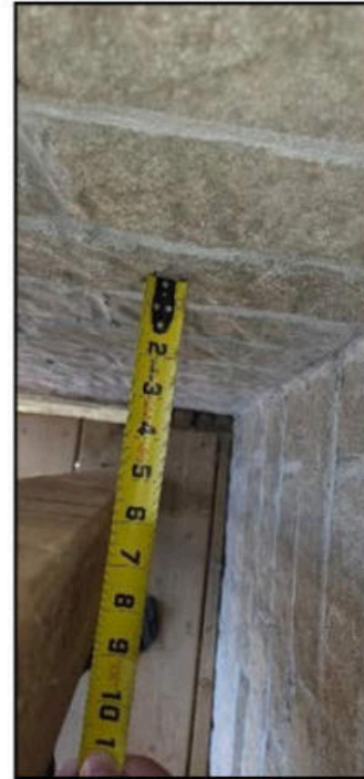
13. Spindles (balusters) too far apart
