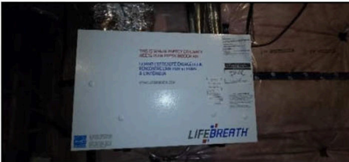
39. Heat recovery ventilator (HRV)
